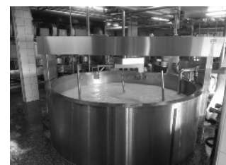
Cuve (local de production).
